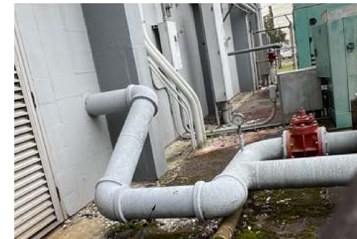
PROPOSE LOCATION FOR CONNECTION OF NEW 3" GAS TAP TO SERVE GENERATORS. COORDINATE SHUT-DOWN OF GAS SYSTEM WITH OWNER. MODIFY EXISTING PIPE AS REQUIRED.
